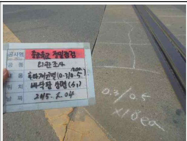
A1 Rail Joint 후타재 균열
